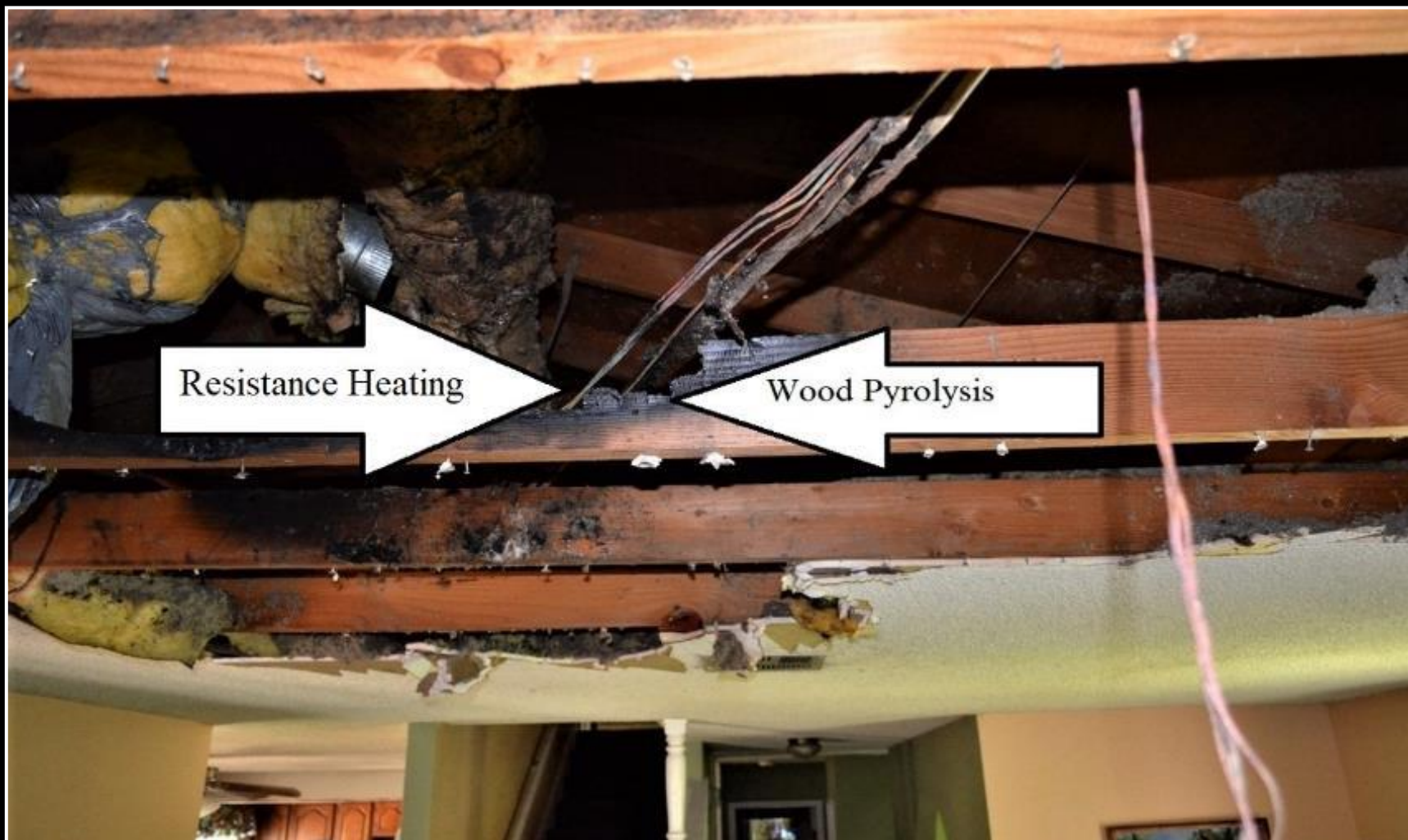
Typical Fires Resulting From Wiring Breakdown
